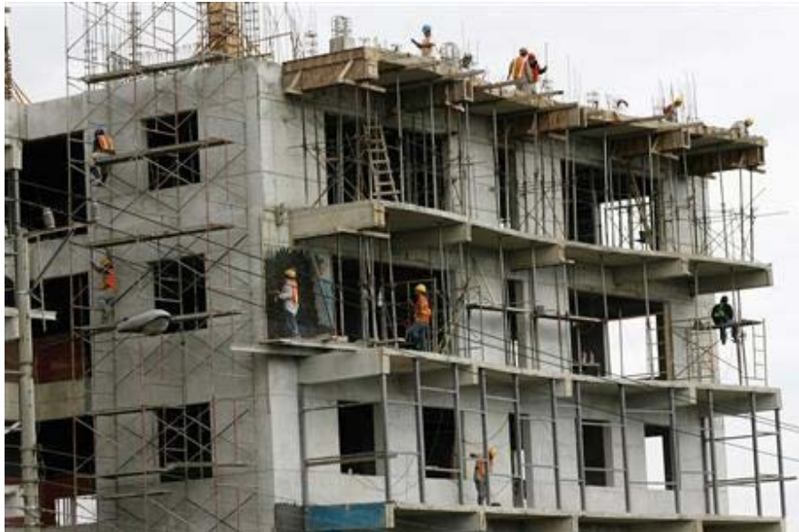
Workers are pictured at a condominium construction site in Santa Ana west of San Jose, August 1, 2008.
